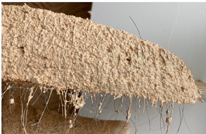
Image of properly haired base coat of plaster. Approx one hair every 1/8 of an inch.
